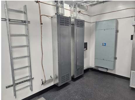
Inside of the Armag modular A.R.C. vault shelter with its MPE Extended Performance TEMPEST power line filter installed on the back wall
