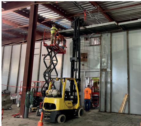
New control centre for power transmission operations serving Midwest USA
