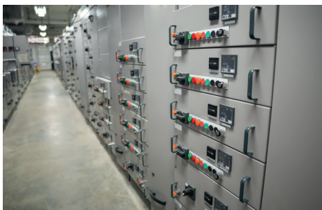
MPE's HEMP protection filters are installed in a US Navy power plant on East Coast USA.
