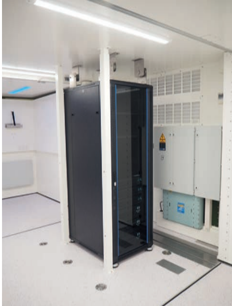
Mobile datacentre with 32A MPE power line EMC filter installed
