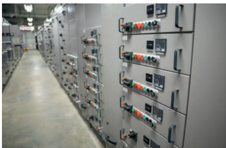
MPE's HEMP protection filters are installed in a US Navy power plant on East Coast USA.
