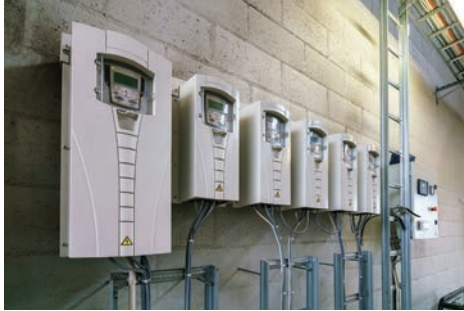
Array of variable frequency drives in situ
