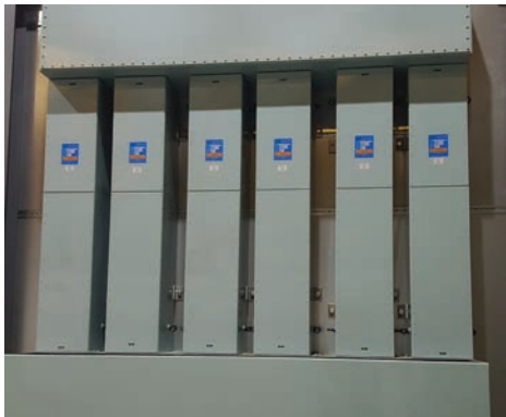
MPE high-current power line filters mounted onto an EMP shield
