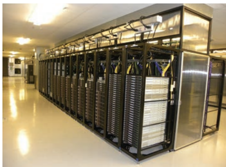
Data centre application typical globally
